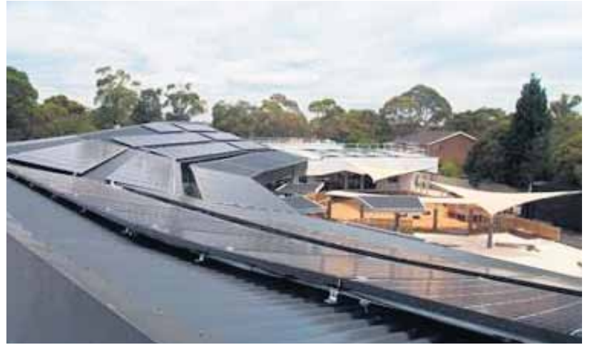
Solar Panels; Knox Children and Family Centre Wantirna South
